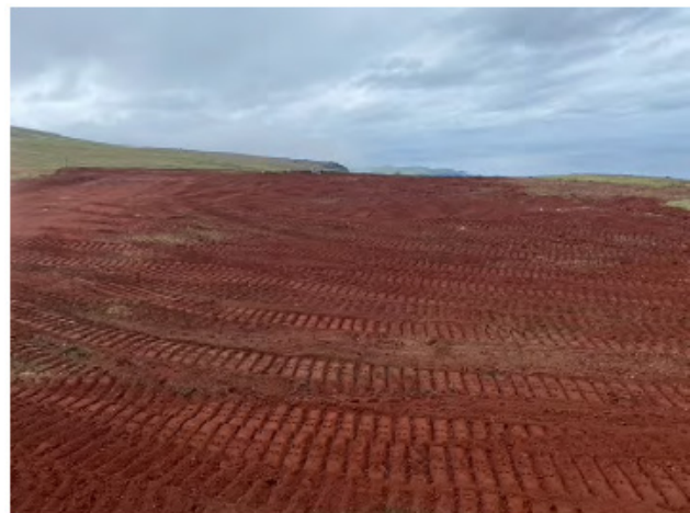
Description: Cap material spread and graded along southern portion of SS02 (Facing west). (6/17/22)
