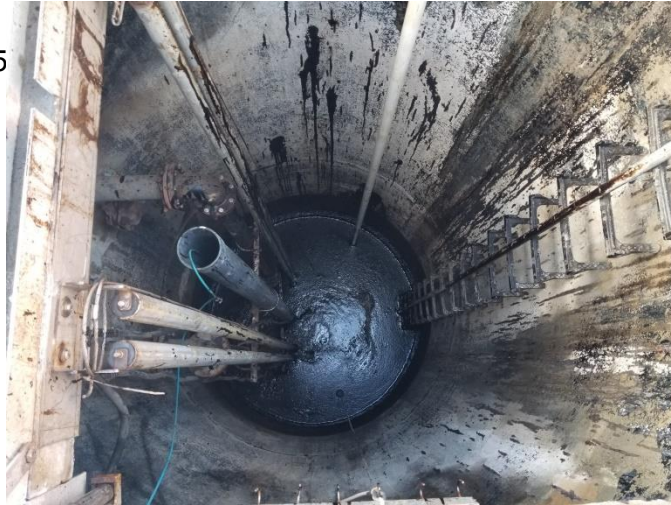
Sewer Lift Station – Oil Contaminated
