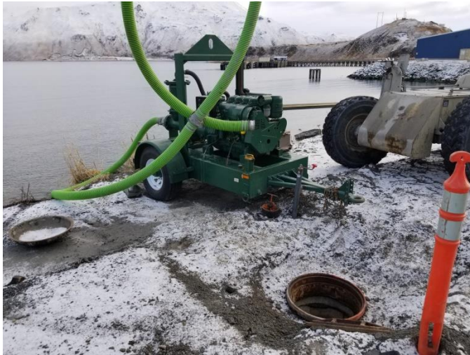
Sewer Bypass Pump
