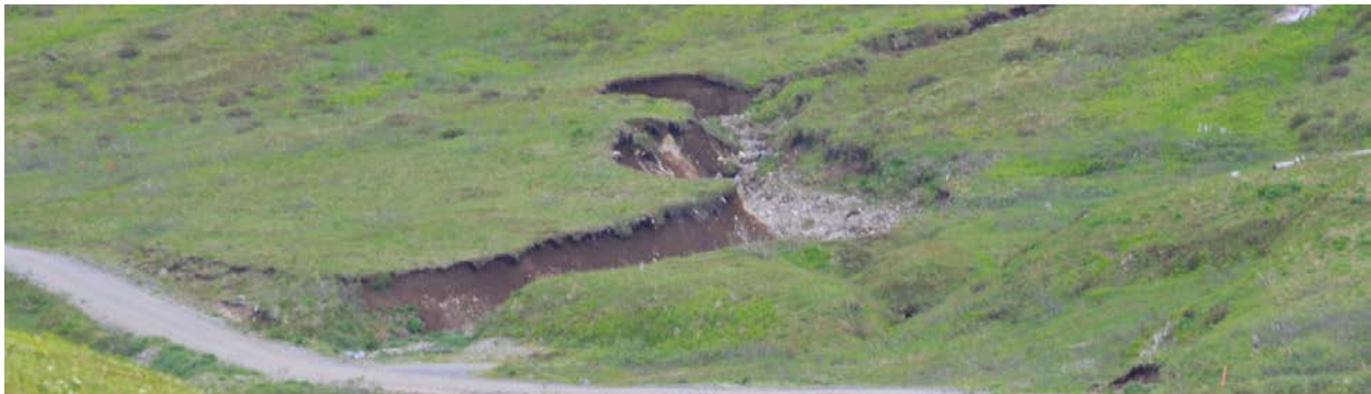
Photo 8-6. Steward Road Unalaska Valley Area Channel Erosion (photo courtesy of Abi Woodbridge)
