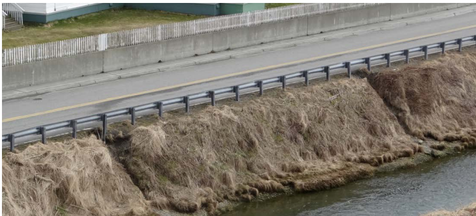
Photo 3-2. Erosion from Runoff Threatening Roadway
