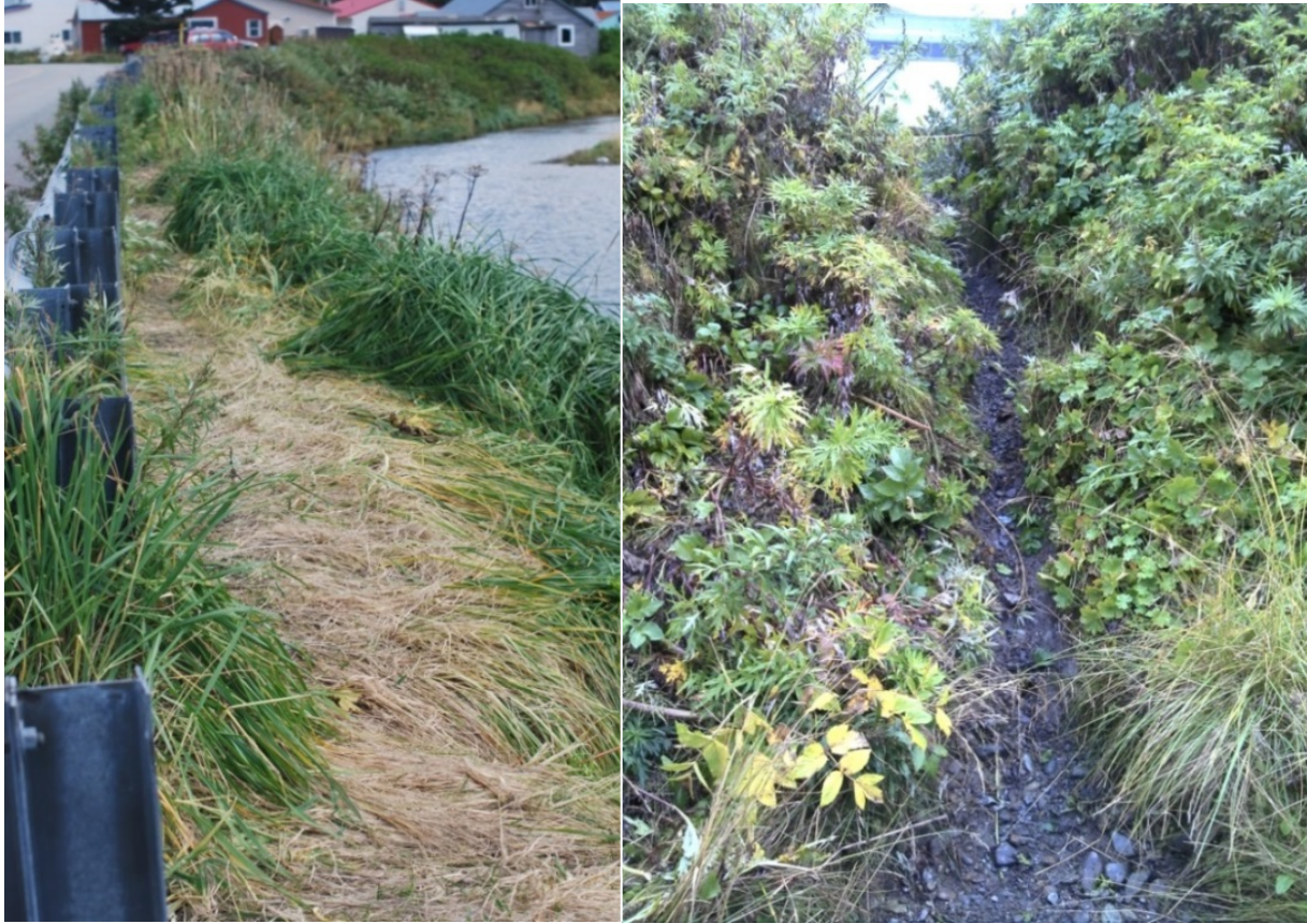
Photo 2-2. Left: Trampled Vegetation along Guardrail; Right: Noted Erosion on Upper Riverbank due to Surface Drainage
