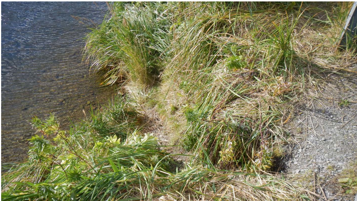
Photo 2-3. Noted Erosion along the Banks of the Lower Iliuliuk River due to Foot Traffic
