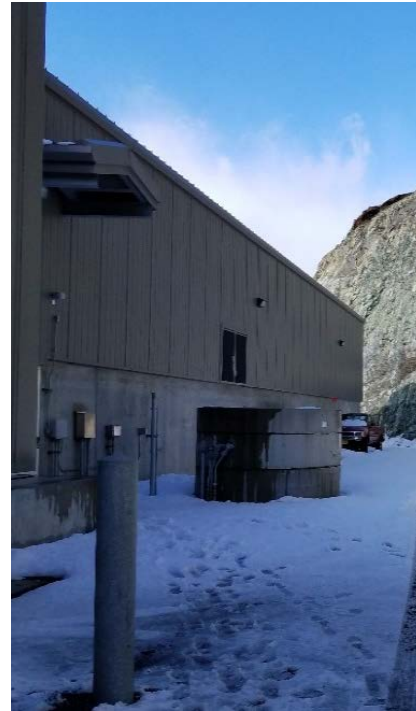
Figure 5-4. Photo of Tank Drain Pump Station
