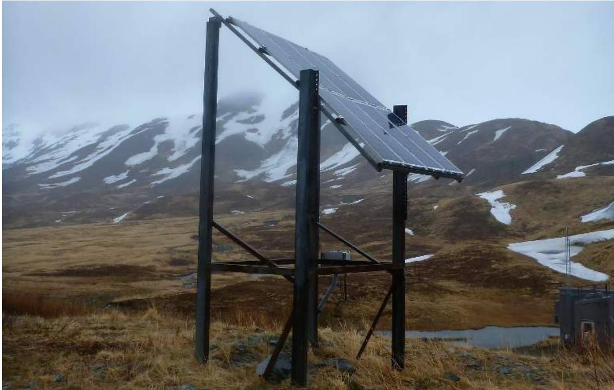
Figure 20: Existing Solar Panel Array at Icy Lake Valve Station
