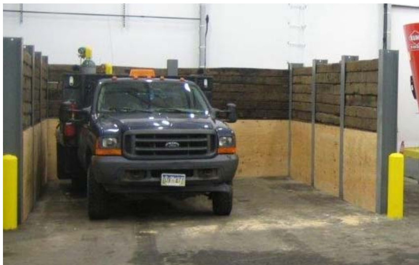
Figure 3. Biosolids Receiving Bunker with Wooden Walls
