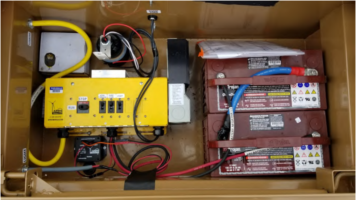
Obstruction light batteries and turbine controller
