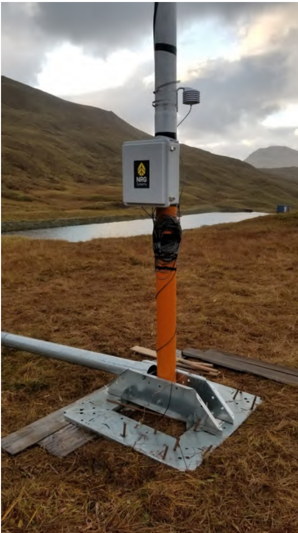
ICR 34 m, tower base
